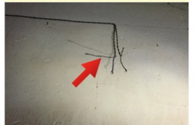
Abandoned Wiring, Remove
