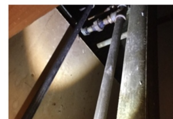
More Copper Gas Pipe
