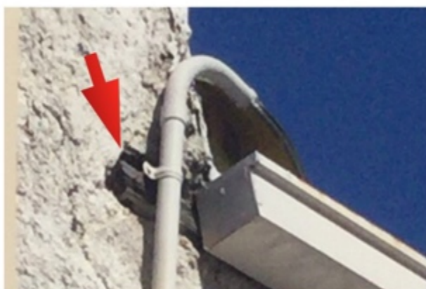
Rotted wood that mast is secured to
