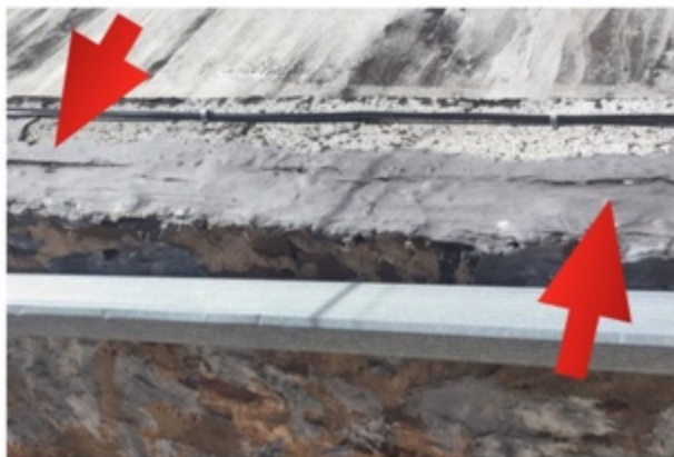
Cap flashing is a tar coating and it is separating in multiple spots
