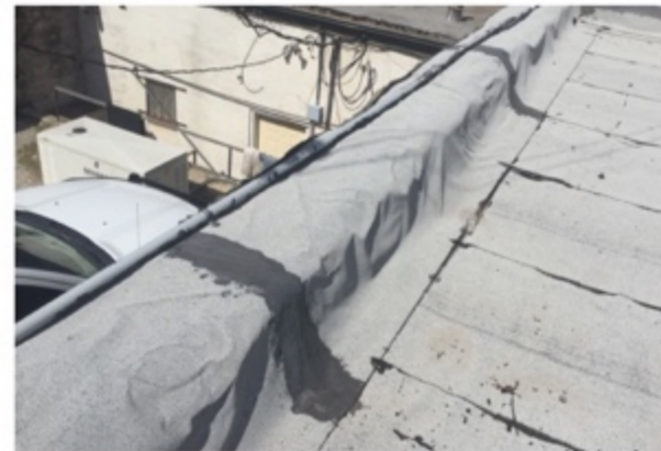
Newer lower N roof. It has several curls and ridges in roll material. It makes it vulnerable for damage and to hail
