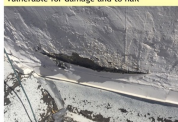
Another opening at roof wall joint. This is over the police building. It can effect this building
