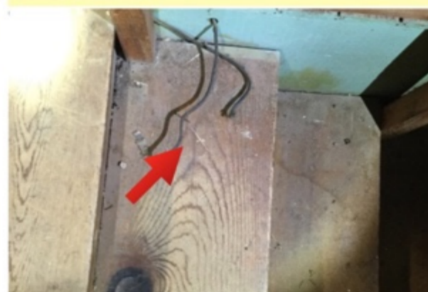
Abandoned Wires At The Stairs
