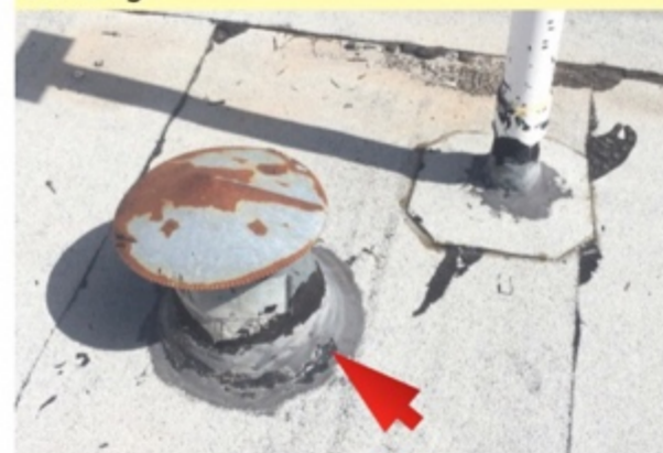
Flashing (tar) is starting to separate
