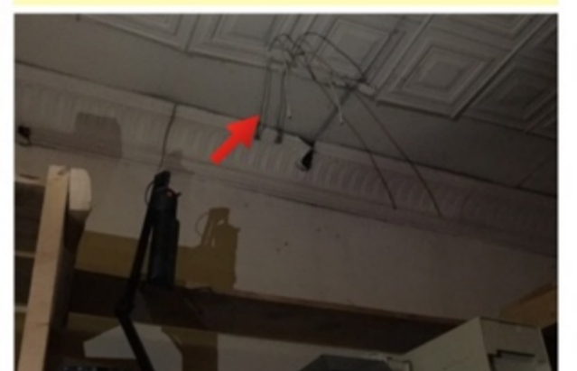
Abandoned Wires Through Ceiling
