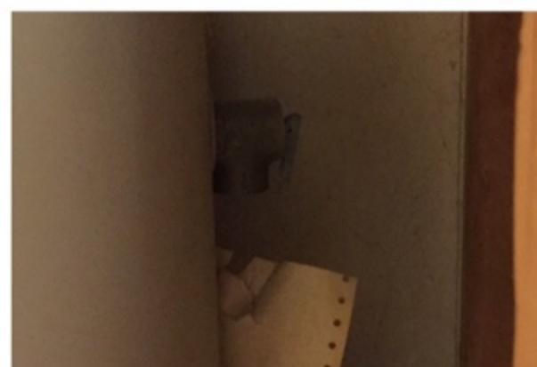
No Pipe At Pressure Relief Pipe
