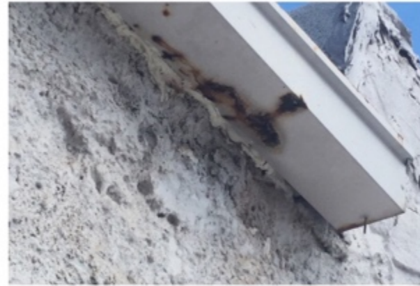
Gutter for upper N. half of the building is rusted through
