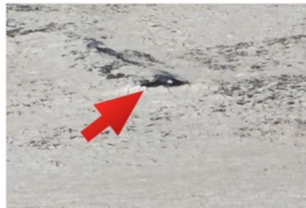
Another unsealed joint/seam in the field of the roof
