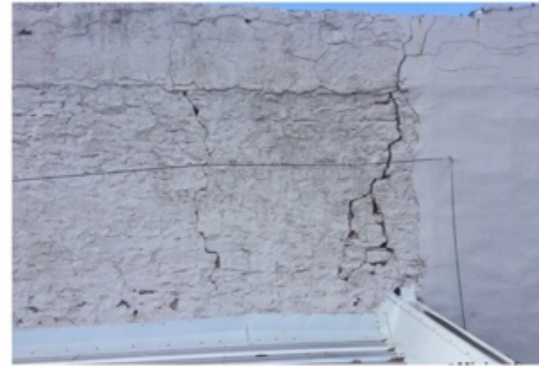
2 of the large cracks on the N. wall
