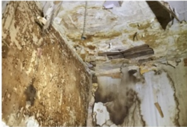
Sever Roof Leak
