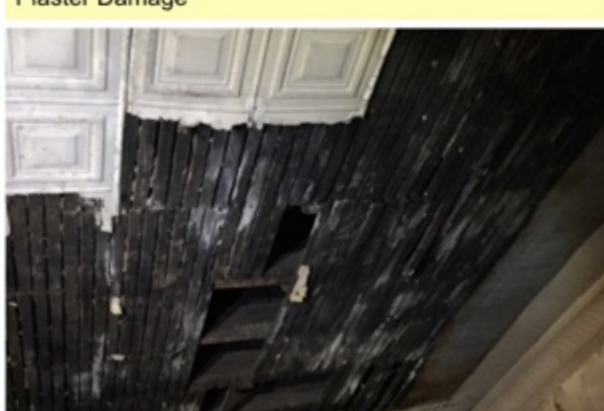
Fire Damaged Ceiling
