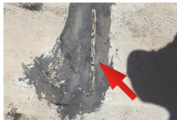
Old patch is starting to open back up
