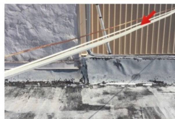
Damaged Romex For Siren Wiring Replace Wiring
