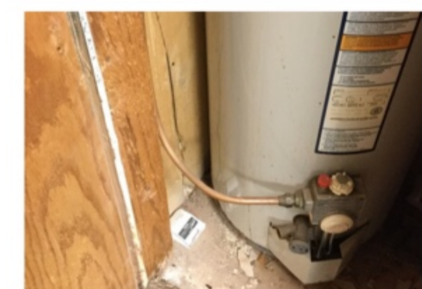
Copper Gas Line
