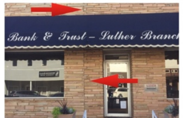
The joint between the N. and S. Sections of the building is cracked all the way up
