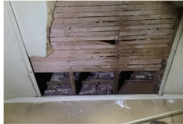
Plaster And Lathe Damage
