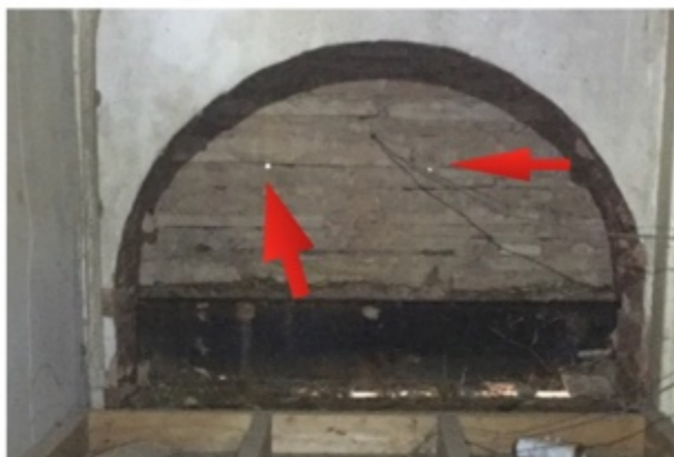
Holes through the front stone work
