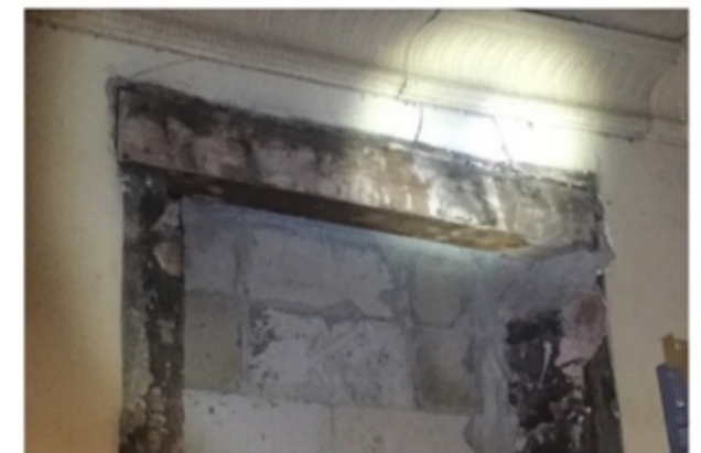
Lintel over old back window is sagging
