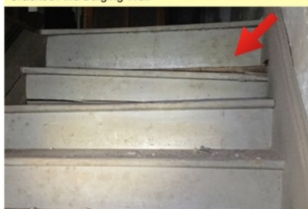
2 Stairs Are Damaged At Top
