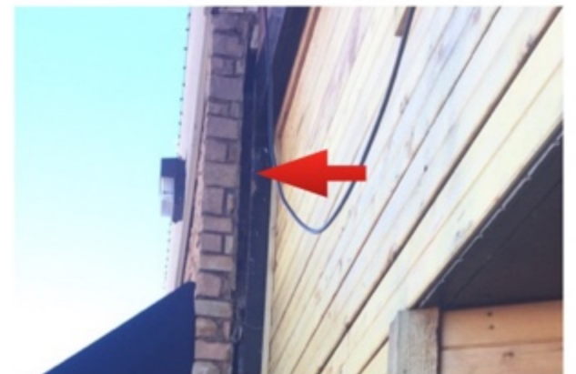
Front stone work is pulling away from the building
