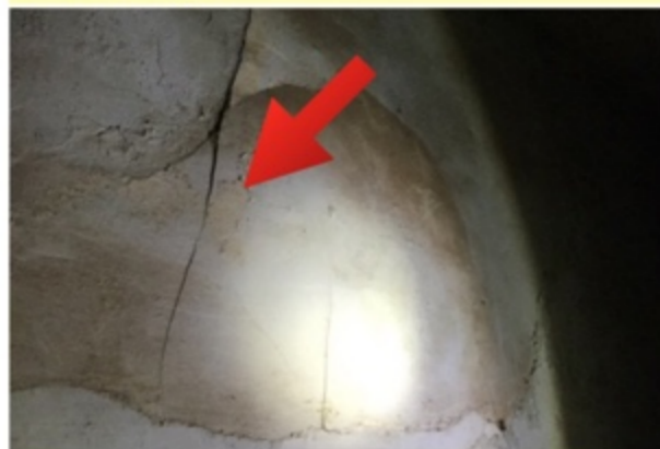
Cracked And Bulging Wall
