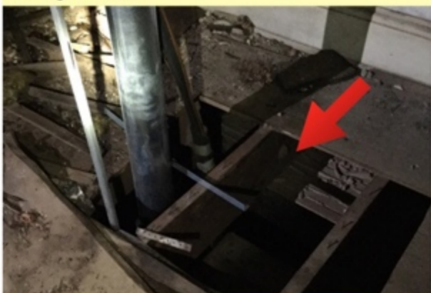
Floor Repairs Needed And Flue Enclosed If Used
