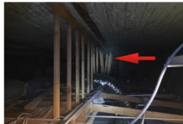
Support for drop ceiling of the N. half. Should be checked during structural eval
