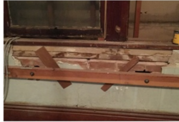
Plaster And Lathe Damaged, Supports For Exterior
