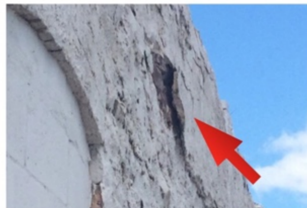
Stucco on the N. wall is starting to fall off
