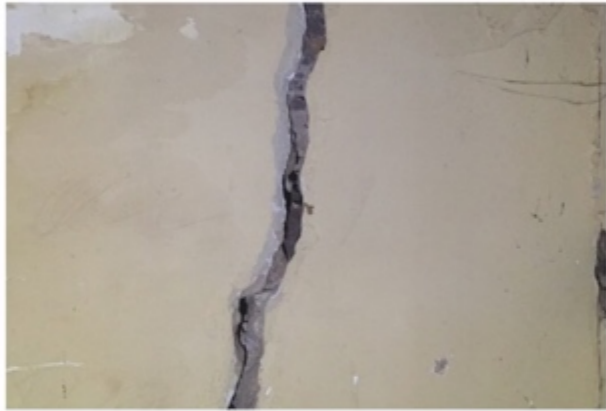
Large crack inside on the N. wall of second floor
