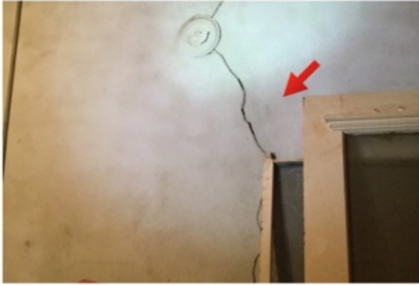
Cracks Above Doors
