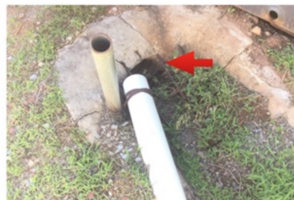
Both gutters of S. Half of building drain into this drainage pipe
