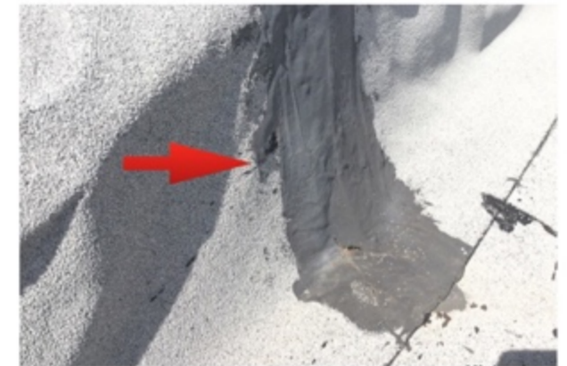
Opening in joints
