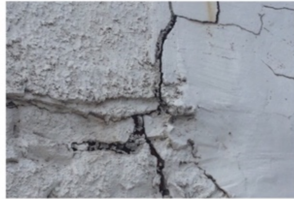
Large crack on exterior N. wall that was sealed & now reopened
