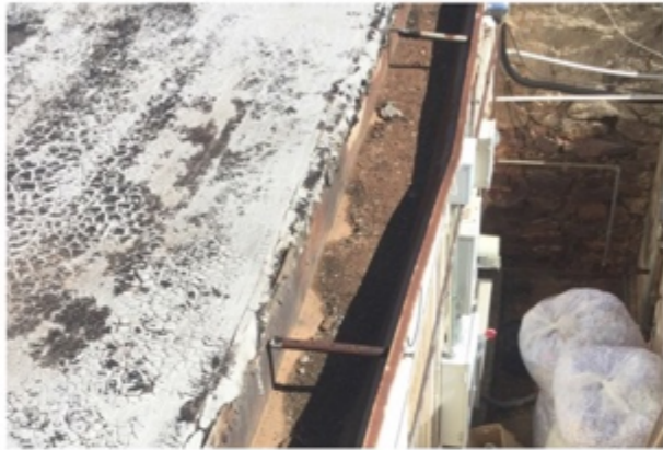
Gutter at back of lower S. Half is damaged and full of debris
