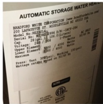
Plumbing Data Plate Breakroom
