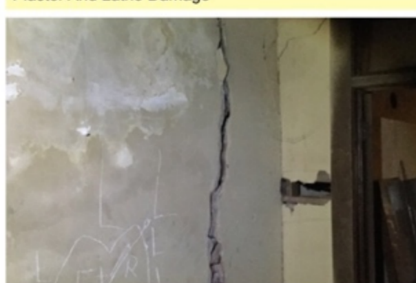
Large Crack To Wall
