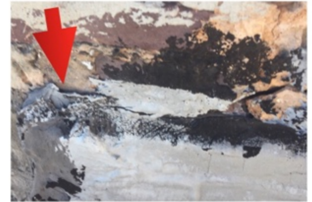
Roof wall joint of lower S. Half is separating
