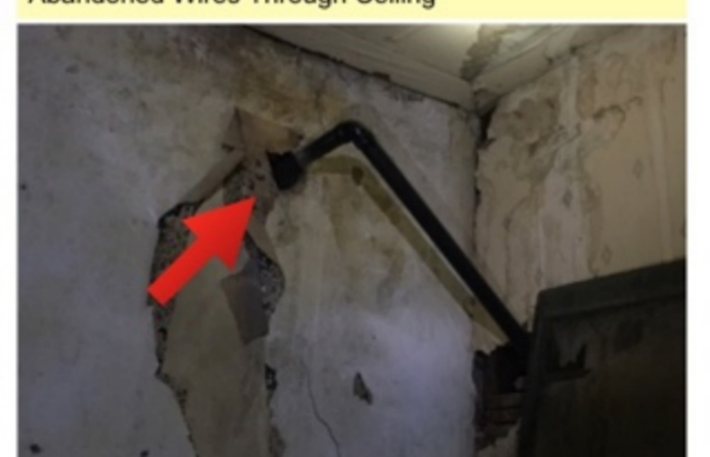
Plumbing Vent Not Venting To Exterior
