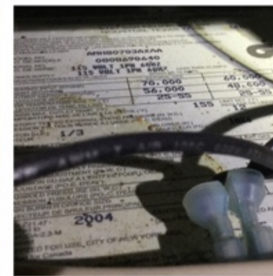
Furnace Data PLate Nw Office Closet
