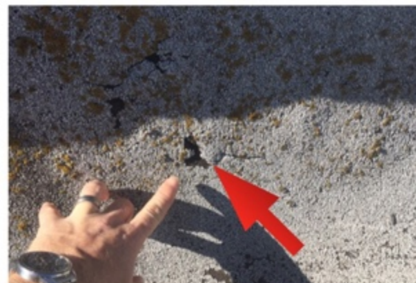
One of the punctures in the roof wall joints
