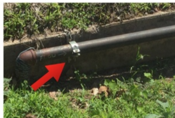
This is the large gas line
