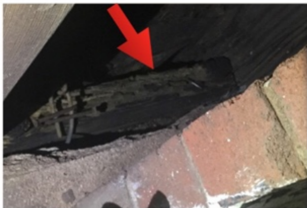
Rotted framing used for siding at front of building
