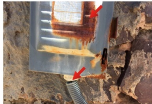
Repair Conduit Break, Paint To Keep From Further Rust
