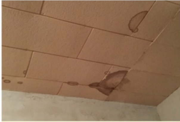
Water Staining In Ceiling Tiles
