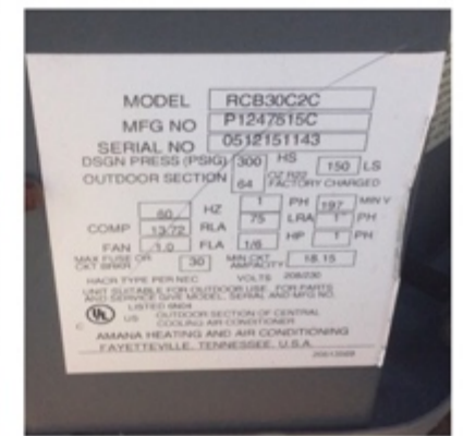
Furnace Data Plate Roof Closet
