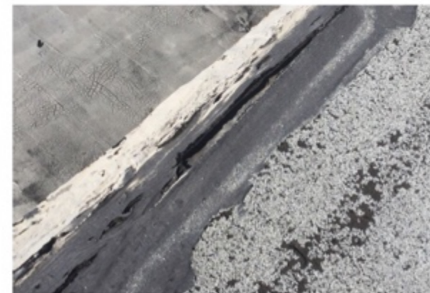
Separation at the upper level cap
