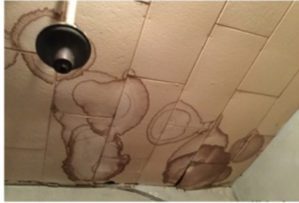
More Water Staining
