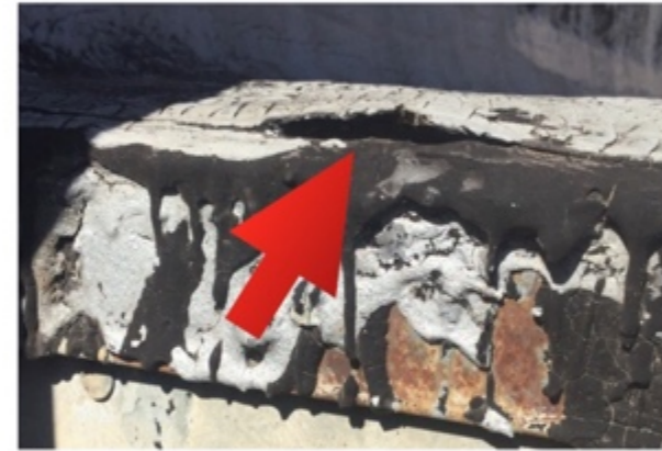
Joint in roofing not fully sealed
