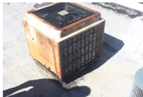
Old unit just left on the roof. It should be removed
