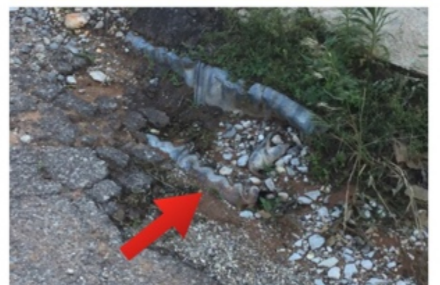
Drainage pipe is crushed at the other end
