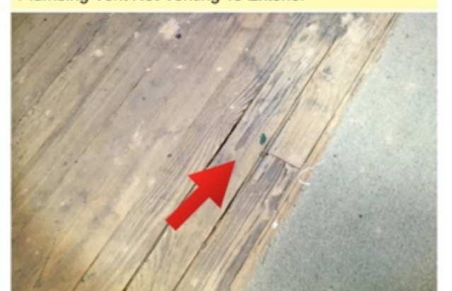
Floors Are Soft In Spots
