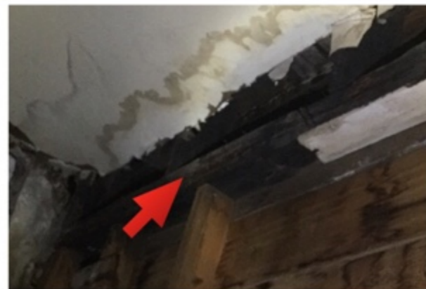
Rotted framing visible from second floor
