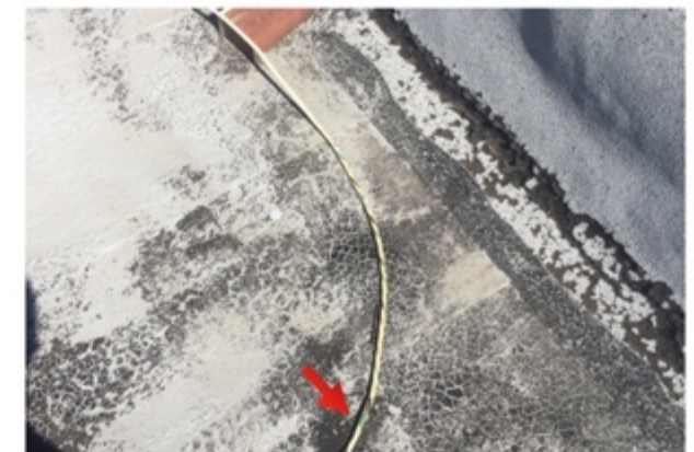
Damaged Section Of Extension Cord
