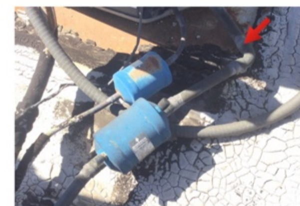
Replace Suction Line Insulation
