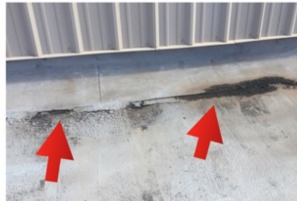
Joints are separating in roofing materials
