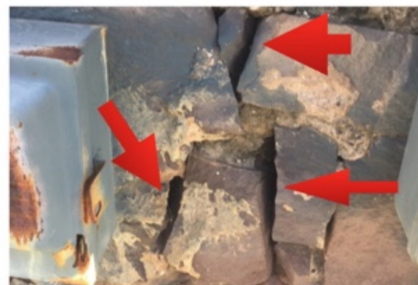
Some of the gaps in the exposed sections of stone work
