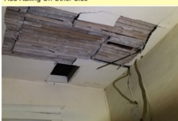
Ceiling Plaster And Lathe Damage
