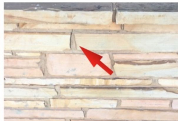
Crack under front window
